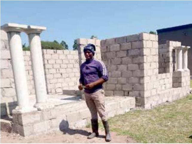
Sabelo Zungu joined ACAT's programme in 2025. Attending ACAT training has made him to develop more love for assisting other people in his area. It motivated him to start a construction business, building houses (above) by so doing he is supporting his community while providing for his family
